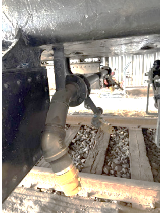
Trackside fill piping
