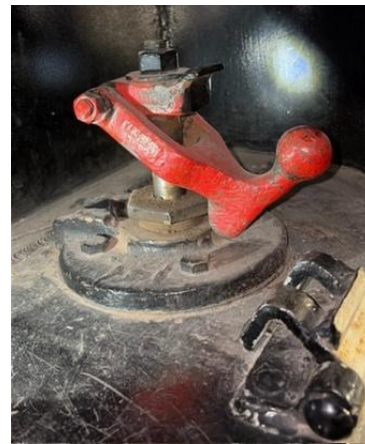
Cold water pump inlet valve
