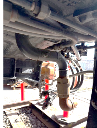
External canteen piping
