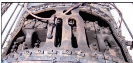
Superheater manifold looking forward
