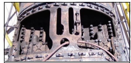
Superheater manifold looking backward
