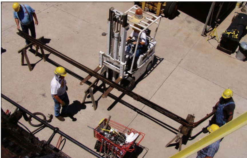
Superheater pipe is moved by forklift to a workstation for cleanup. Photo by Mike Harts-horne from top of 2926.
