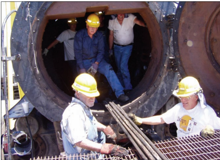
Milestone is reached, but much work left: Guided by McEntire, Ormson and DeGroft, the first superheater pipes slide forward from smokebox onto scaffold.
