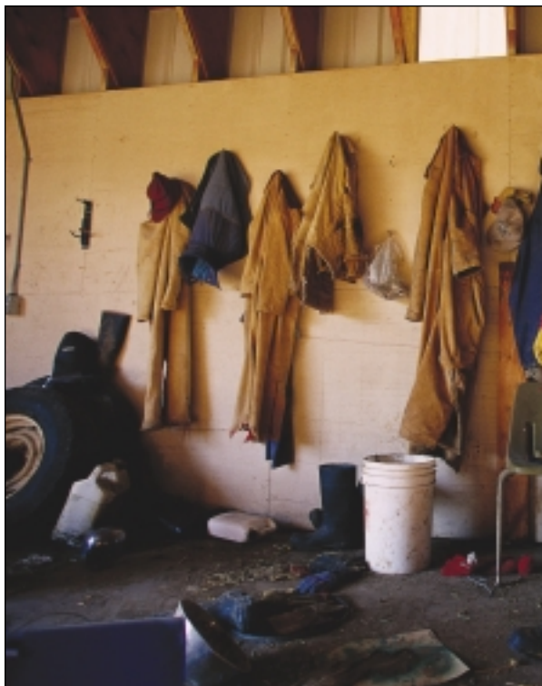
This barn presents a clear fire hazard. Maintaining a clean barn free of hanging cobwebs, loose hay and straw, compressed gases, clothing, and cleaning supplies is excellent fire prevention and requires minimal daily effort.
