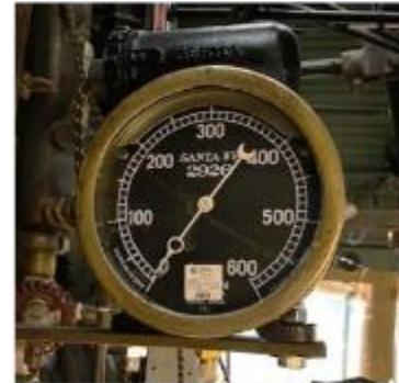
Main steam pressure gauge
