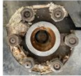
Boiler inlet diffuser
