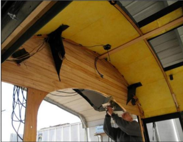
Woodwork in the cab: Pete Ormson uses a power sander to finish the edge of woodwork that is being installed in the 2926 cab.
