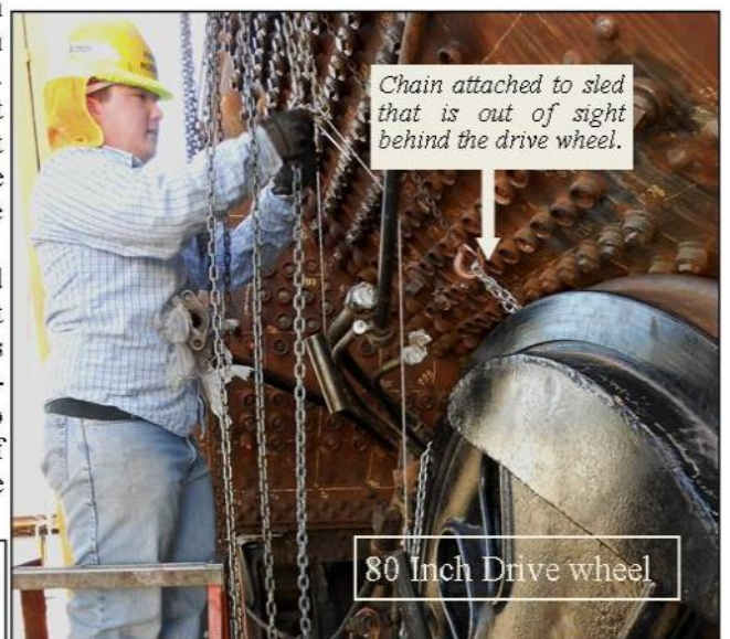
Right: On the fireman's side, Henry works control chains to keep tension on the chain attached to the sled. The sled is holding the wrenchito and box wrench on the staybolt cap. A similar arrangement is on the engineer's side.
