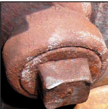
Cap Closeup: A half century in place, and tightened by corrosion.
