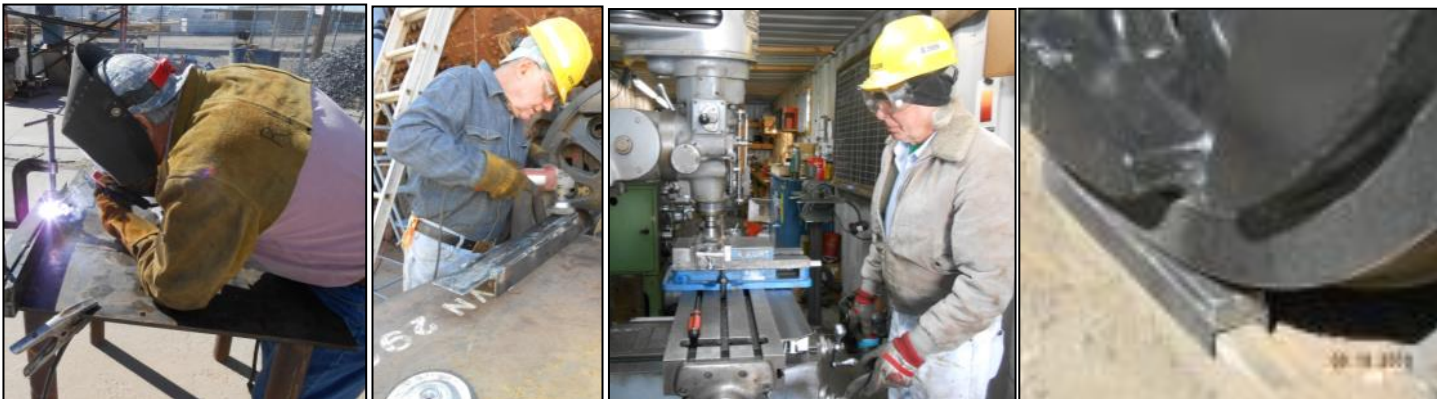
GOT TALENT? This is how the 2926 team works—with a bit of basic common sense guidance from a retired steam era pro. At Glen Powers suggestion, Rick Kirby, Dave Van de Valde, and Ron Taylor make short work of fabricating the wedge pictured in use in the last photo.
