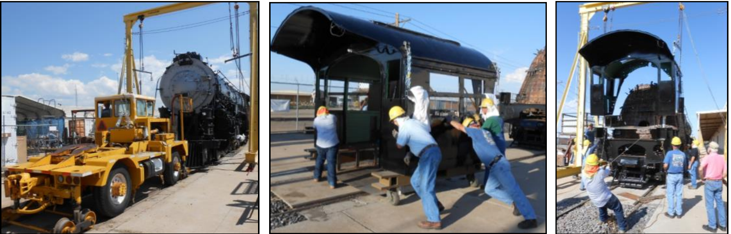
Left: Car Mover ‘Lurch’ pulls 2926 westward next to the GSA warehouse to clear ‘Big Bird’, the gantry crane. Center: Volunteer muscle power moves cab (mounted on a dolly) to the tracks at the rear of the locomotive. Right: After repositioning ‘Big Bird’, more muscle power is applied to hoist and steady the cab as 2926 is nudged under the cab by Lurch. With a lot of jiggling and tugging, the cab is then eased into place.
