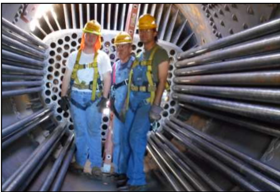
It's a start! The inside team, Henry, Martin, and Anthony stand inside the boiler next to the rear flue sheet at the start of the flue tube insertion. Their job was to take the tubes pushed to them by the smokebox team, pull them through the boiler, and feed them into a matching rear sheet hole. Most tubes pictured are the smaller ones. The space in which the team is standing grew smaller and smaller as additional tubes were inserted. The last tubes at the very top were guided through by the workers either lying in the tight space above the tubes or reaching through from the manway 'entry hatch' on top of the boiler.
