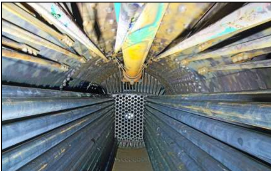
Inside The Heart Of The Beast: Photo art by Ron Taylor. This image was produced by processing seven exposures into a single image using High Dynamic Range software. The view is from a top center flue tube hole in the front flue sheet, looking to the rear flue sheet at the firebox. The cluster of bright spots in the center of the rear flue sheet is natural light entering through the open firebox door on the cab side of the firebox. Copies of this and other examples of Ron's digital art, merging old steam and new digital technologies, and suitable for framing, can be purchased at the 2926 Site Store. Proceeds go to the completion of the 2926 restoration.
