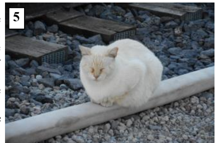
5 Cat Waterbed? For some reason, the feral cats living on site like to sit on the fire hose. Several have been spotted on hoses, especially when the hoses are full of water while filling the boiler.
