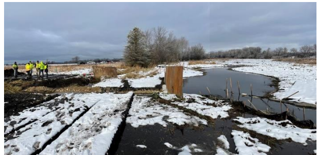
Before “tie in” of new channel with original channel: road plates divert water away from sensitive areas through a diversion channel.
