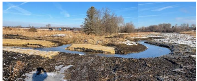
After “tie in”, the completed stream course flows through the area right to left.
