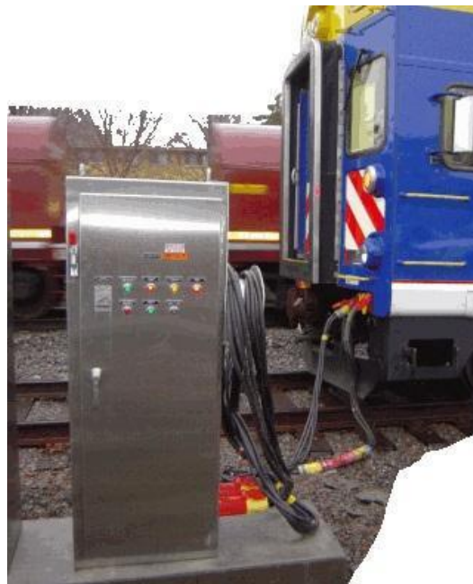
480 VAC shore power device
