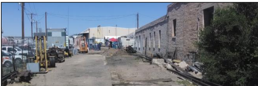
Track Repair, Looking West From 8th St: Siding repair will limit restoration work and visitor access until about the end of the month of May. The locomotive and tender were moved west toward 12th St, next to the GSA warehouse.
