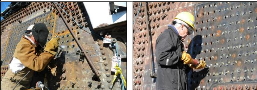
Beginning a two year saga: January 2012, staybolt reinstallation begins. Staybolt work begins on large patch that was made to the fireman's side of the boiler. The patch was necessary due to corrosion. The original staybolts were also severely corroded.
