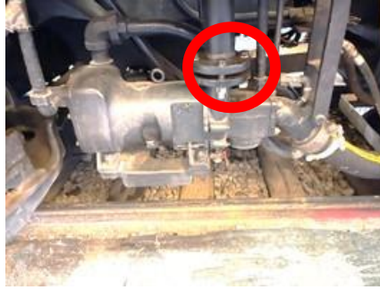
Cold water pump defrost lines
