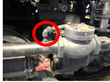
Check valve defrost line
