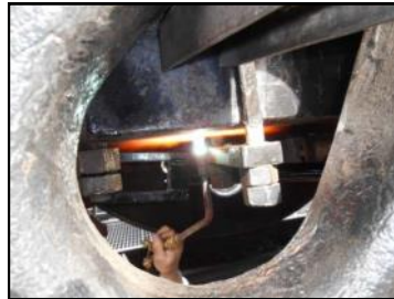
I: Heating pedestal binder bolt as seen through drive wheel.
