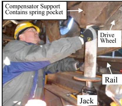
A: Lowering compensator support. In the pit working next to the drive wheel.
