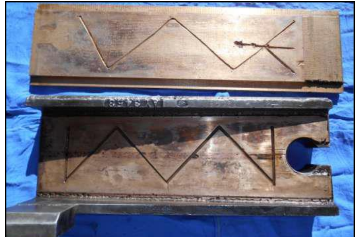
L: Wear Plate (top) and wedge (bottom) show lubrication grooves and little wear. Gap on right end of wedge is slot for wedge bolt head.
