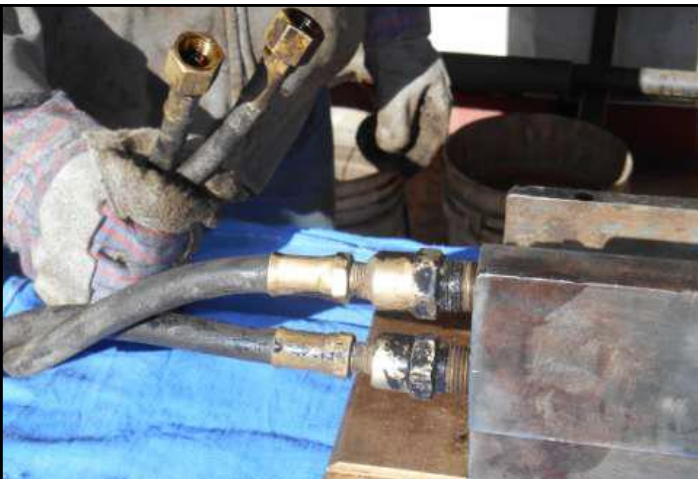
K: The 2926 "modern" lubrication lines attached to the top of the wedges provided a learning opportunity for the pit rats.
